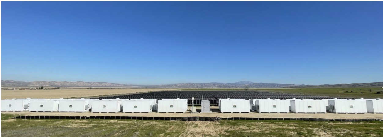
B2U's SEPV Cuyama facility in Santa Barbara County, CA (Operational since Nov 2023)
