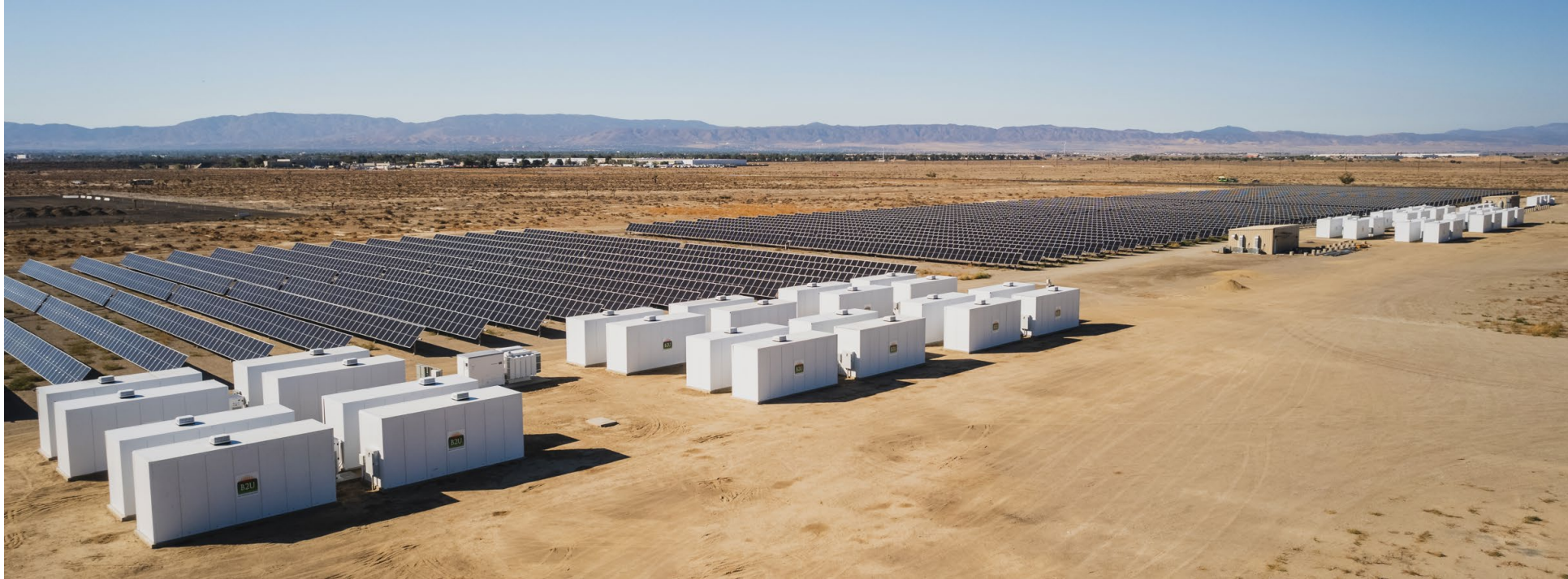
B2U's energy storage facility in Lancaster, CA
