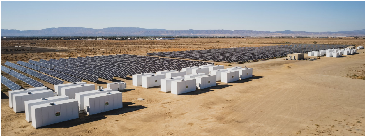
B2U's SEPV Sierra facility in Lancaster, CA (Operational since April 2020)
